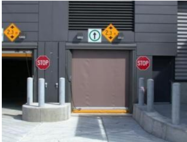
Typical baggage room vehicular entrance – as seen from the Head of Stand Road. Note: Directional indication, 2.3m height clearance, stop sign.
